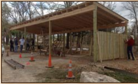
Cart and bike shelter being built by the men of Sunnybrook Church, Stillwater, Oklahoma.
