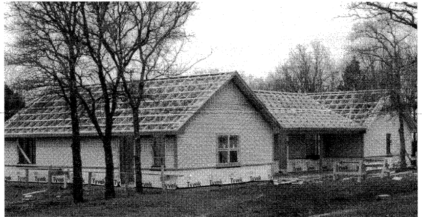
Gabriel House, under construction, will be home to Robert, Mike and one other Rancher, as well as to Amy (Resident Assistant) and husband Eric, the Horticultural Assistant in the greenhouses. Currently, they all live in the smaller Camp Center.
