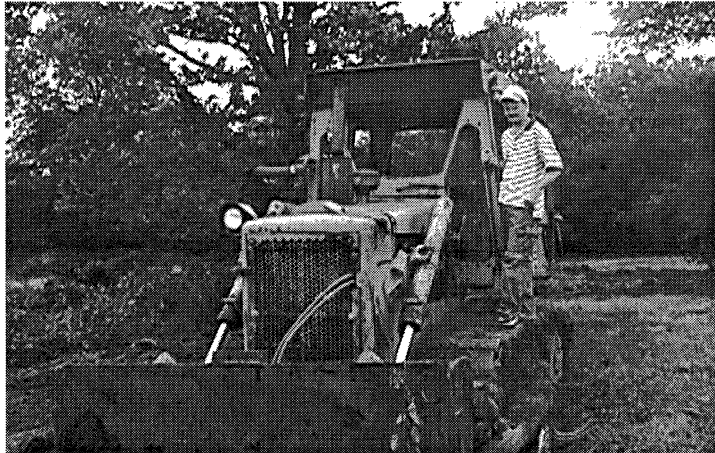
Daniel and Michael on the dozer as clearing begins for The Village—the residential community at Down Home Ranch. The Village road will be a half a mile long, winding through 10 wooded acres. The D5B dozer is on loan from Steve Stoecklein's construction company.
