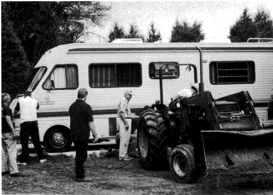
Men from Hyde Park Baptist Church, Austin, auger post holes as part of a project to put a protective roof over Charlie West's motor home. Charlie is donating the home to Down Home Ranch, but will use it for his (we hope) frequent visits to the Ranch.
