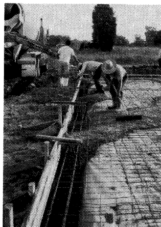
Concrete slab and beams are poured for the Nexus greenhouses donated to the Ranch
