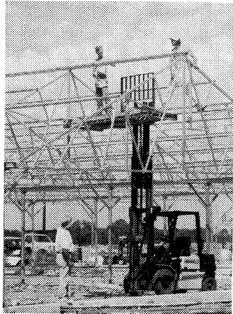
Community service workers from the Bastrop County Restitution Center erect the framework for the Nexus greenhouses
